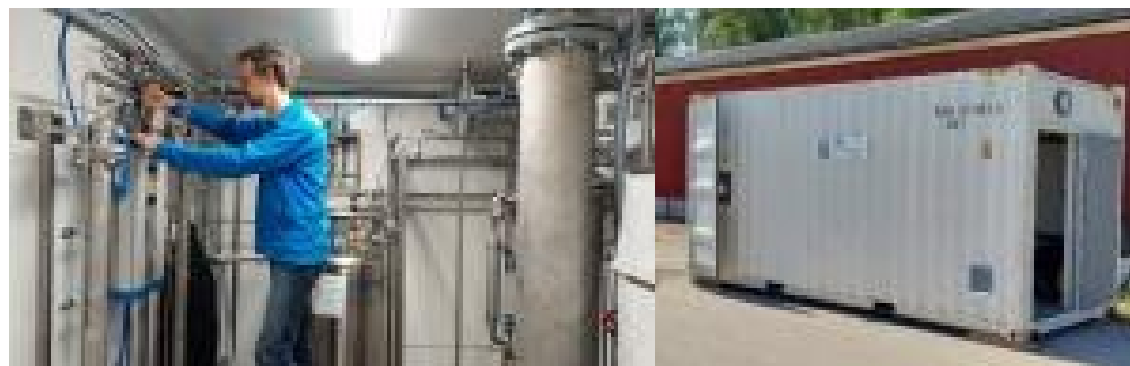
portable gas cleaning pilot plant
