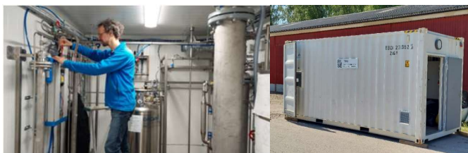
portable gas cleaning pilot plant
